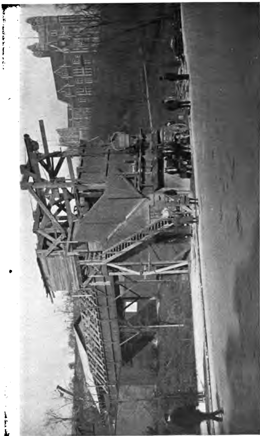
PLATE 213.—Shaft 10. City Tunnel, Catskill Aqueduct. Excavated material is raised at shaft and dumped from cars into bins over sidewalk and hauled away, mostly, in motor trucks.
